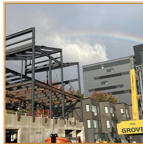
Gladstone Office Extension - New class A office space, rising from the old in the North End of Halifax
